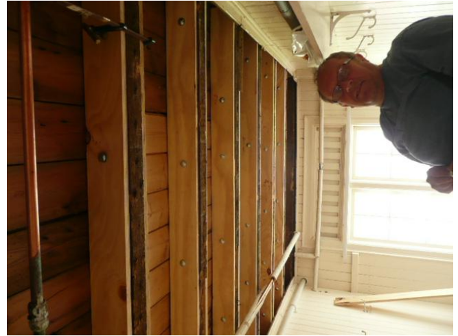
Roger's anti-gravity device came in handy when dealing with the joist re-enforcement. Look at those beautiful bolts...
